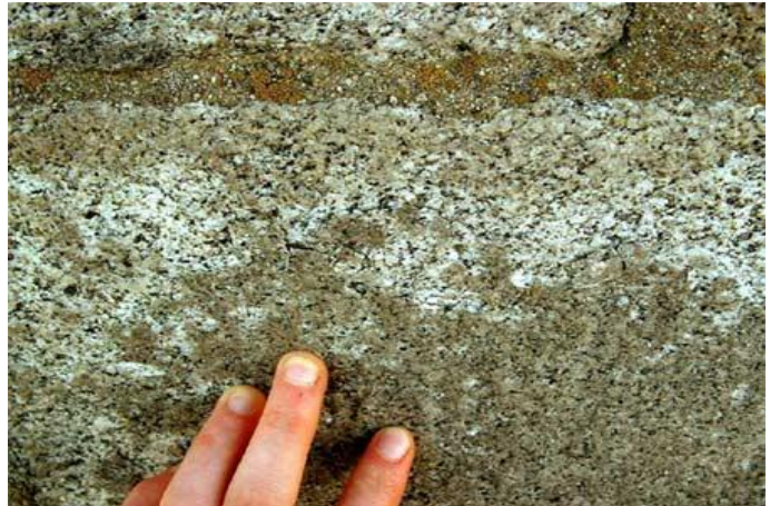
Stone fabric damaged by the effects of salt and moisture.
