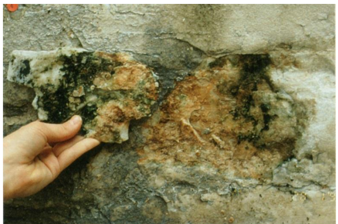
Algal growth on exposed construction elements with a high moisture content.
