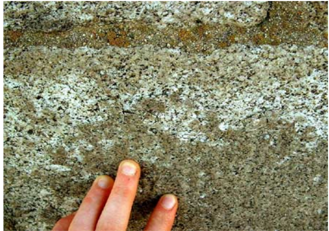
Stone fabric damaged by the effects of salt and moisture.
